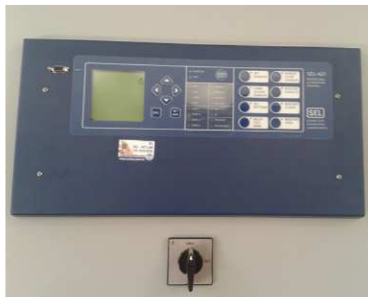
Figura 29: Vista frontal do painel.
