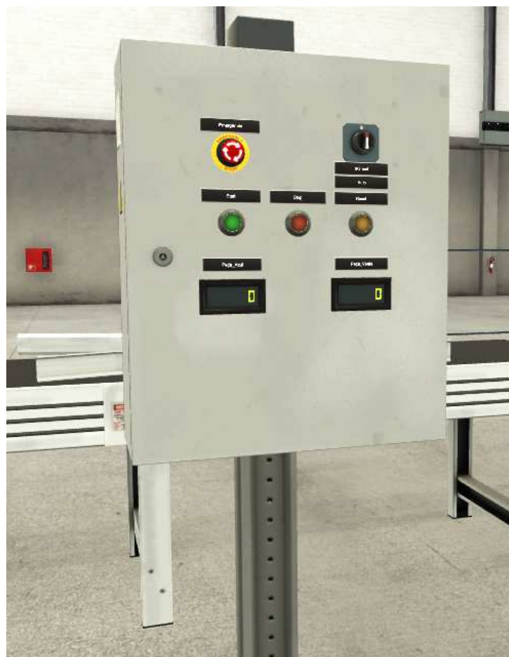
Figura 21 – Painel de Controle.
