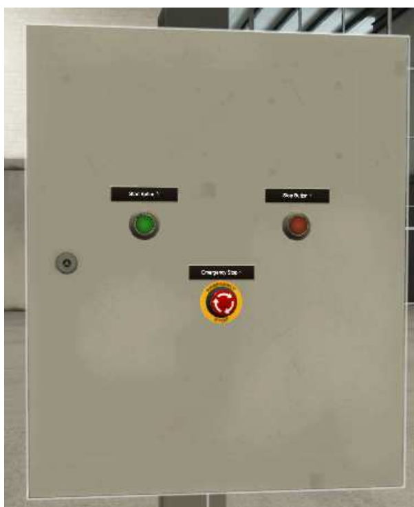
Figura 31 – Painel de controle
