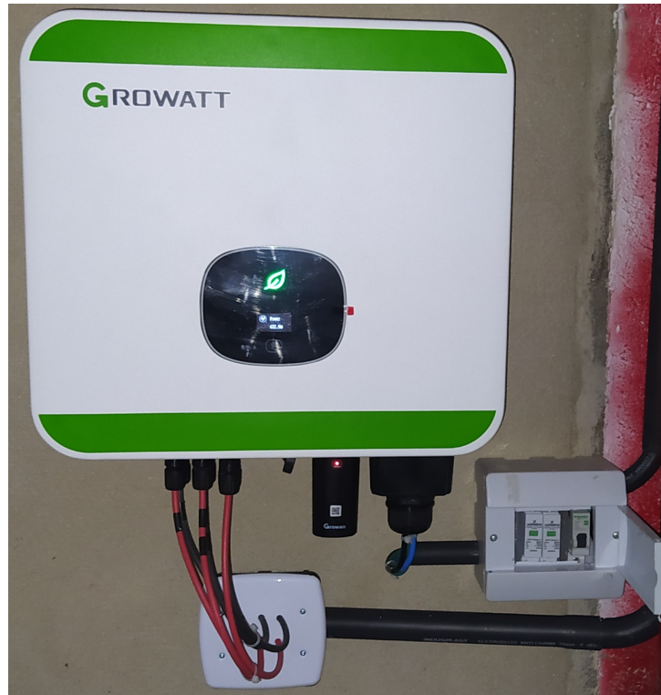
Figura 24 – Inversor Growatt MIN10000TL-X instalado no local.
