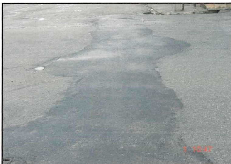
Figura 2.14 – Remendo mal executado (Local: Rua Anacleto Eloy, Campina Grande-PB)
