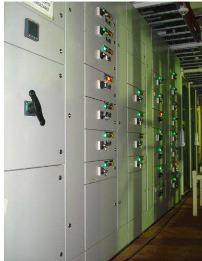
Figura 4.10 – Painel CCM DAS 1.
