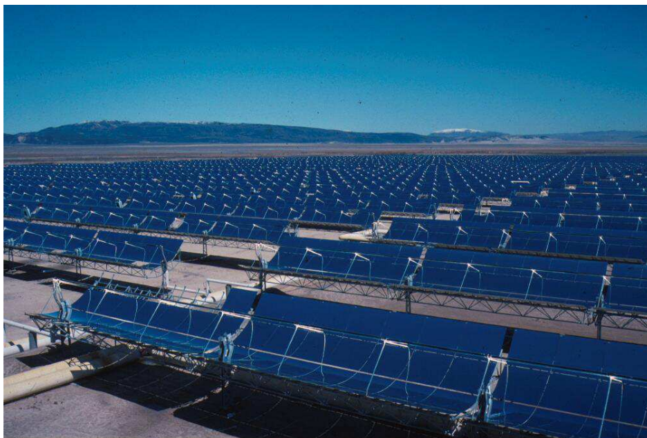
Figura 8 - Solar Energy Generating Systems
