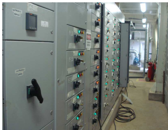
Figura 16 – Vista frontal do Painel CCM FTS.
