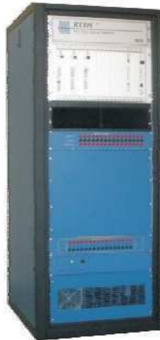
Figura 11: Rack do RTDS™.
