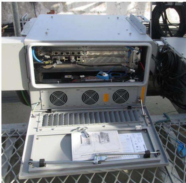
Figura 11 – Nokia AirScale System Module instalado no gabinete FCOB, no site SLRVIL03.
