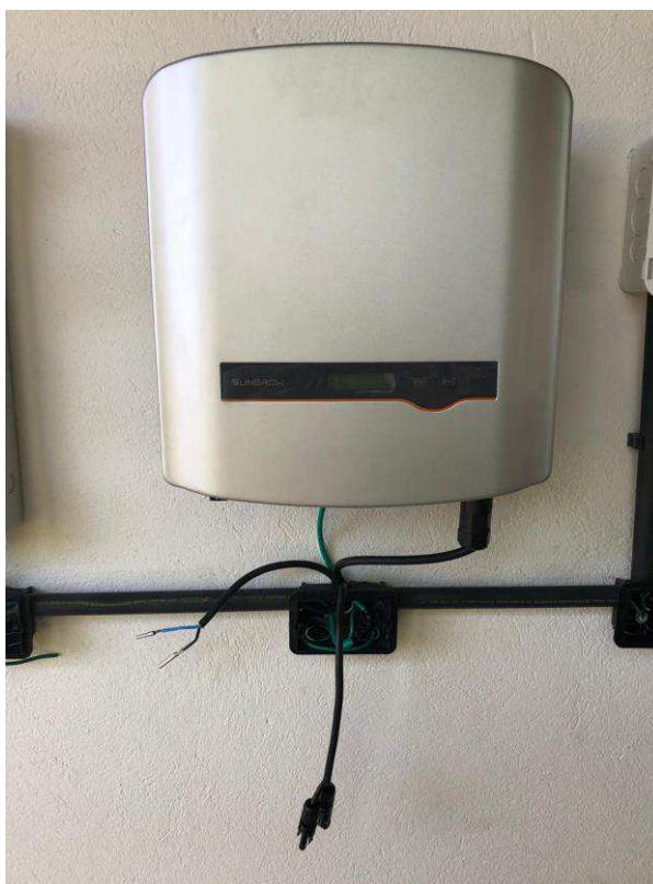
Figura 14 – Inversor da Sungrow.
