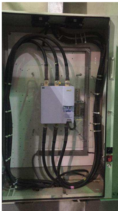
Figura 18 - Painel com soft starter instalada.
