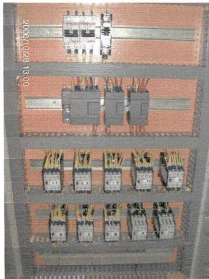
Figura 32 - Quadro do PLC - Programmable Controller System (Siemens)
