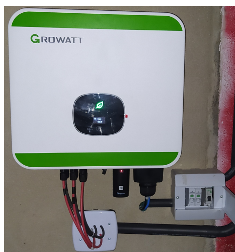
Figura 22 – Inversor Growatt MIN10000TL-X instalado no local.
